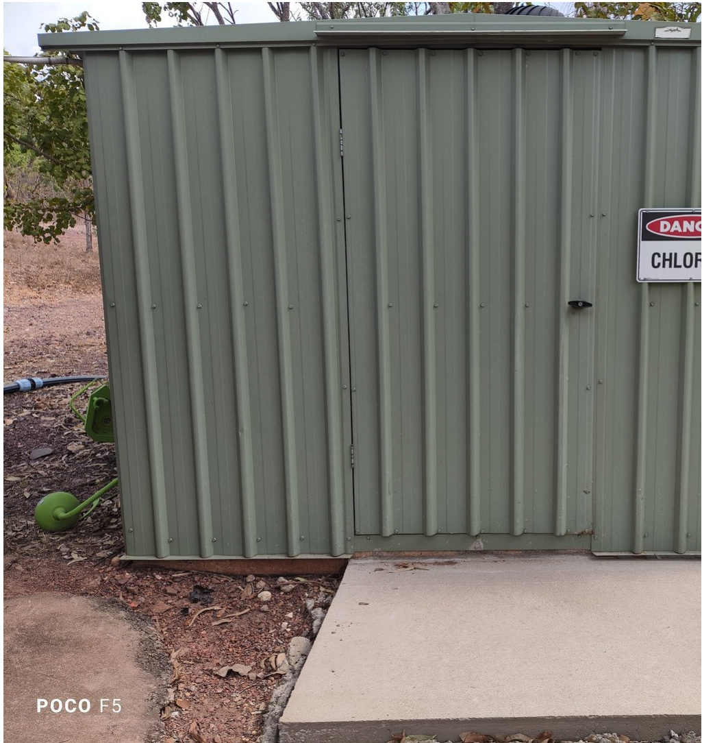
Second Green Shed - Chlorine System - Placeholder
