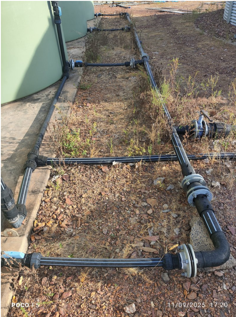
Manifold and Master Valve
