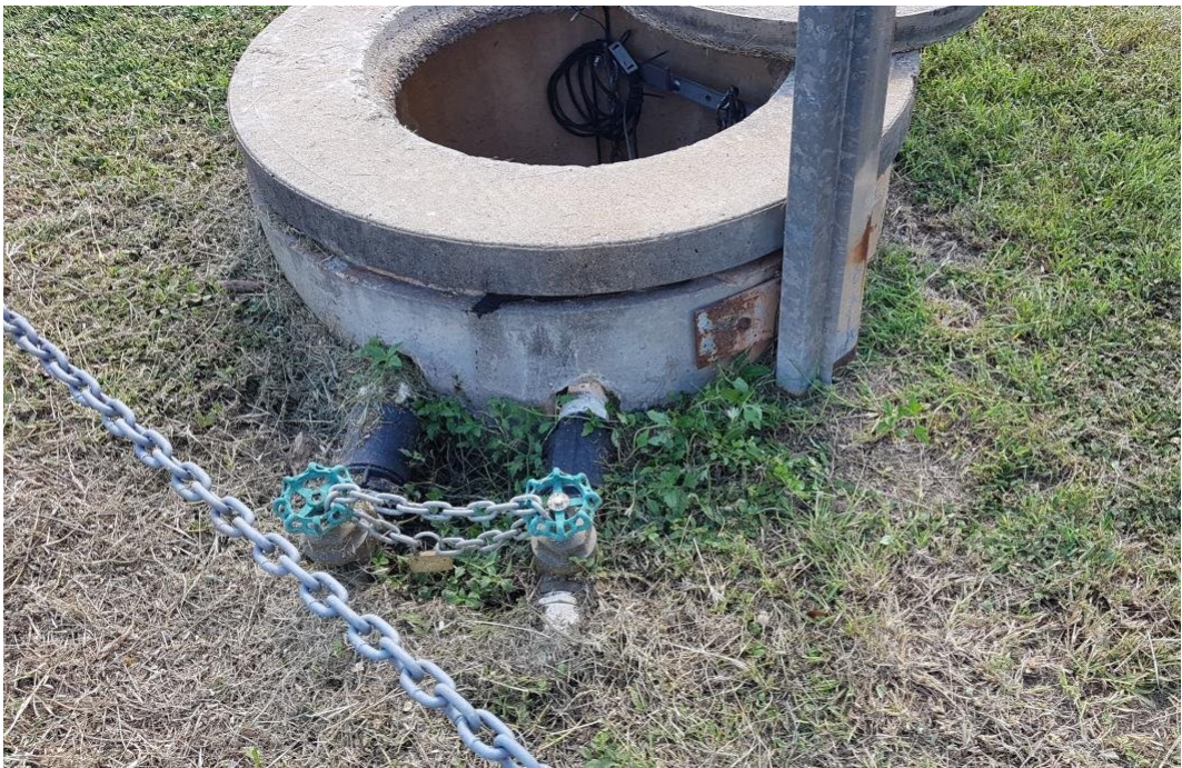
SSP1 Lift well
