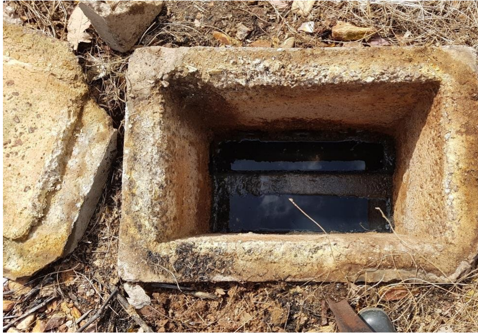
LAA Distribution Box
