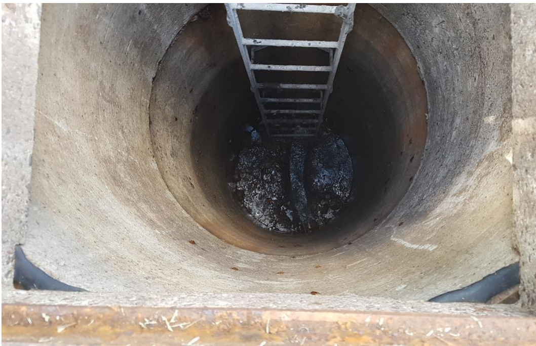
SSPI Large tank Riser 1 - inside
